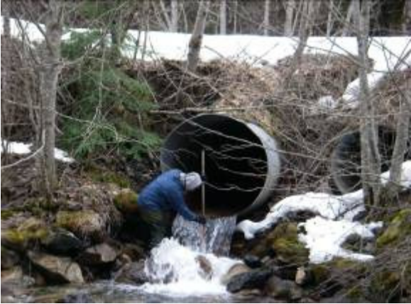
BCCF technician measuring the height of a tributary culvert on Silverhope Creek.
